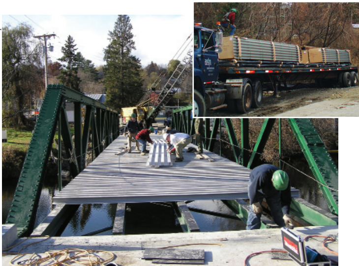
ZellComp's second installation was on an old truss bridge in rural Bradford, Vt. During the November installation, the weather was cold and there was some rain. These conditions would have precluded use of conventional adhesively bonded composite decks or poured concrete. Note that all structural deck components fit on a single trailer truck (top photo).
